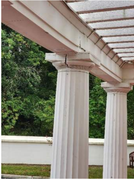
Photograph 7: Column wrap failure.
