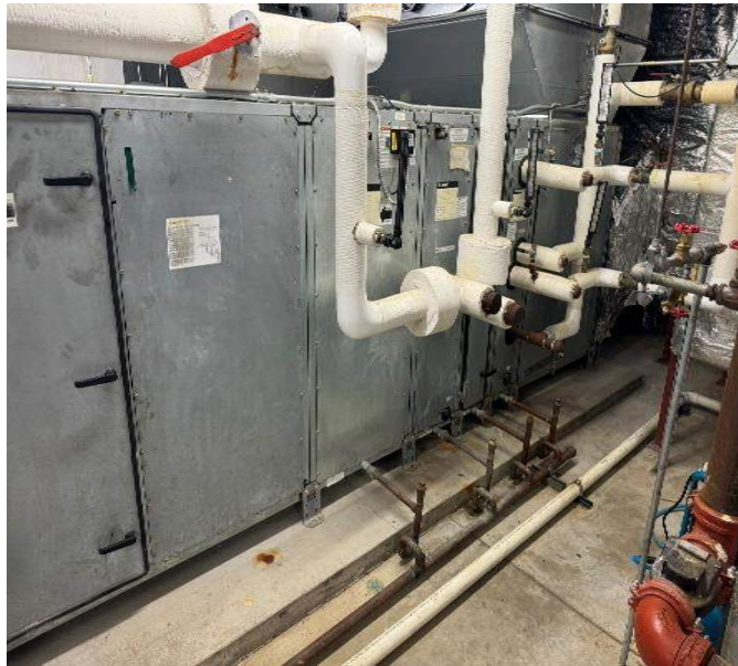
AHU with Chilled Water Coil
