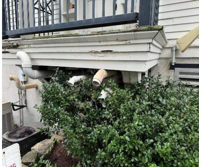
Damage from F/AC Vents
