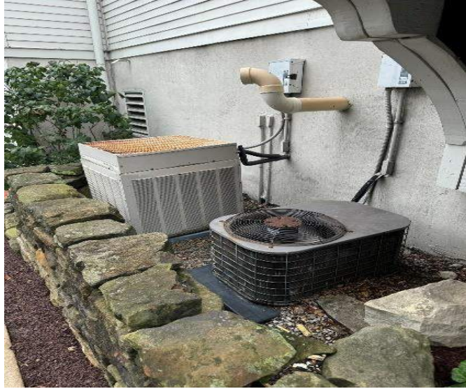
Photograph 2: F/AC Outdoor Condensing Units.
