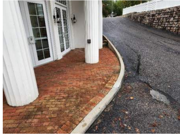
Photograph 5: Absent frost slab at outswinging exterior door.
