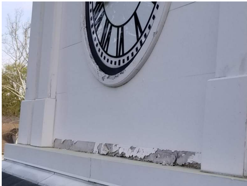
Figure 16: Cupola base trim issues.
