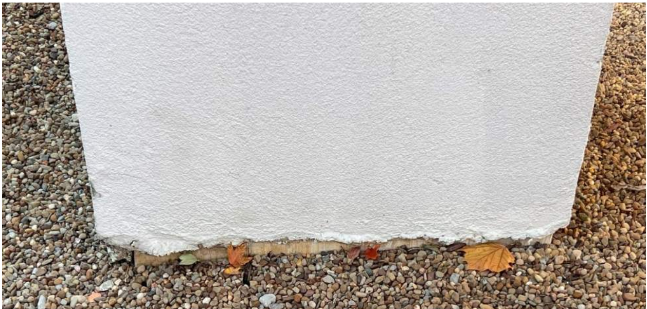
Figure 6: EFIS damage at base of concrete pillar.
