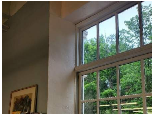
Photograph 14: Gap above east exterior window in the Bookstore Area.
