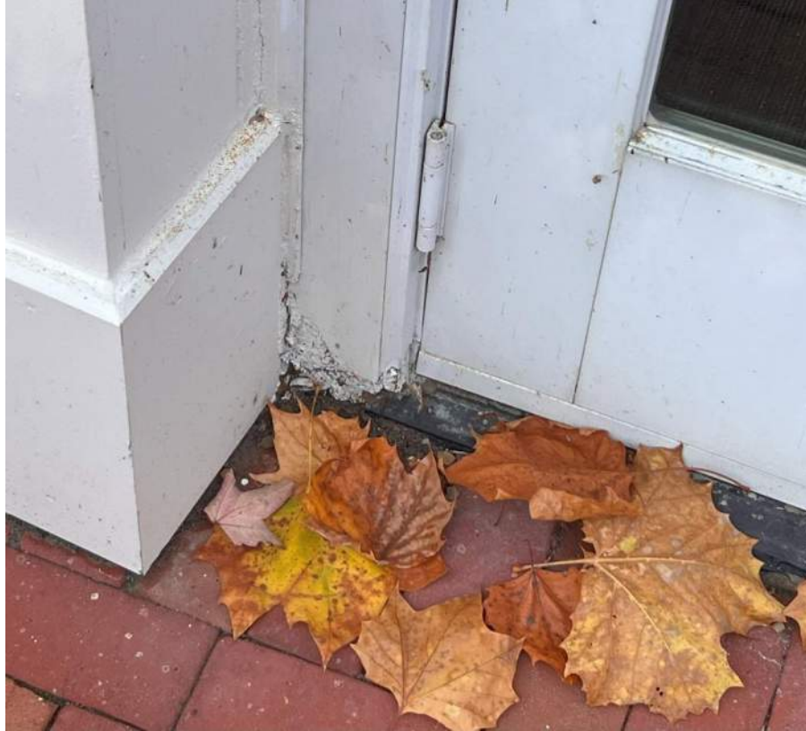
Figure 10: Door trim base rotting at West Elevation.
