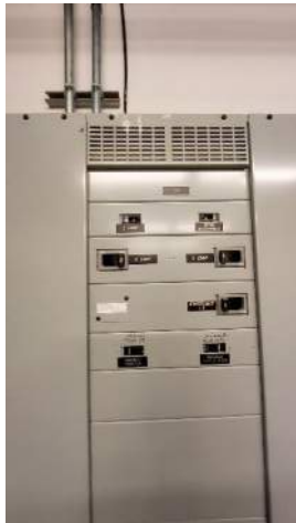
Photograph 21: Main Distribution Panel.
