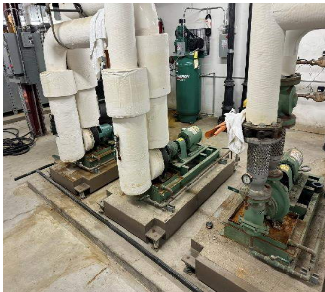
Chilled Water Pumps Coil
