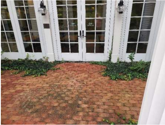
Photograph 4: Absent frost slab at outswinging exterior door.
