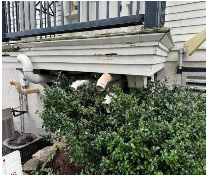
Photograph 3: Damage from F/AC Vents.
