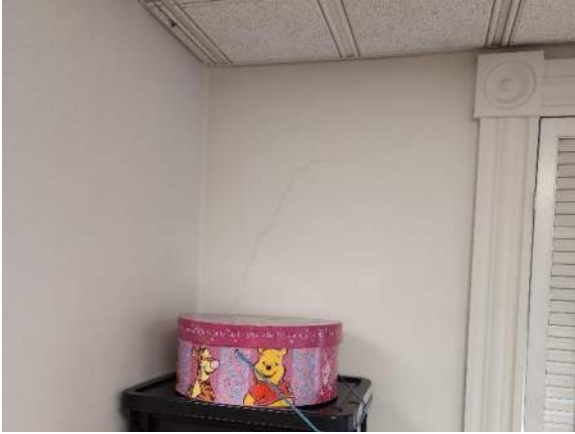
Photograph 23: Cracking in wall.
