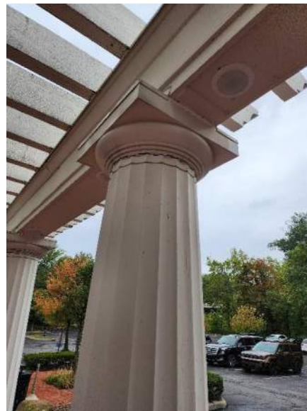
Photograph 8: Column wrap failure.
