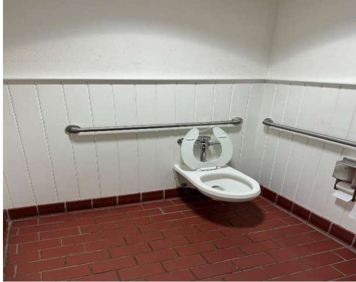
Photograph 13: Water Closet w/MFV.
