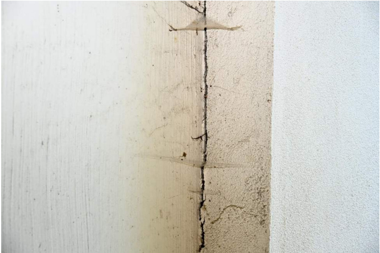
Figure 5: EFIS crack underneath main-level balcony.
