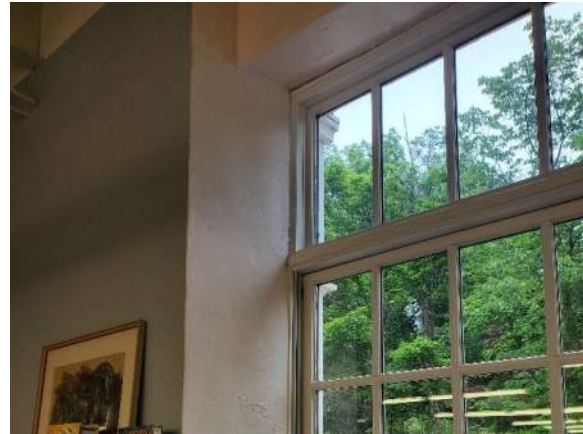
Photograph 17: Gap above east exterior window in the Bookstore Area.
