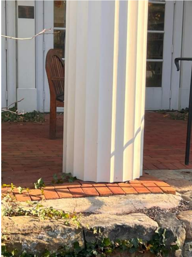
Figure 5: Column base at center patio location. The surrounding paver settlement indicates concrete support under column.
