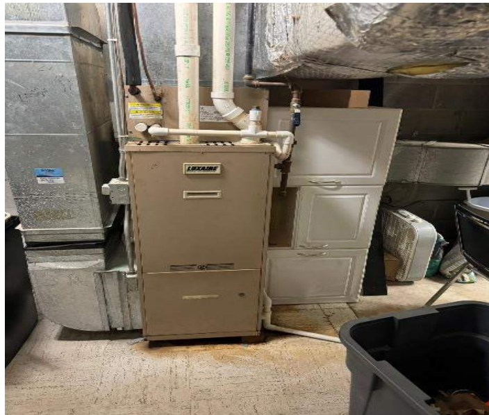
Photograph 8: Furnace/AC Unit (original building).
