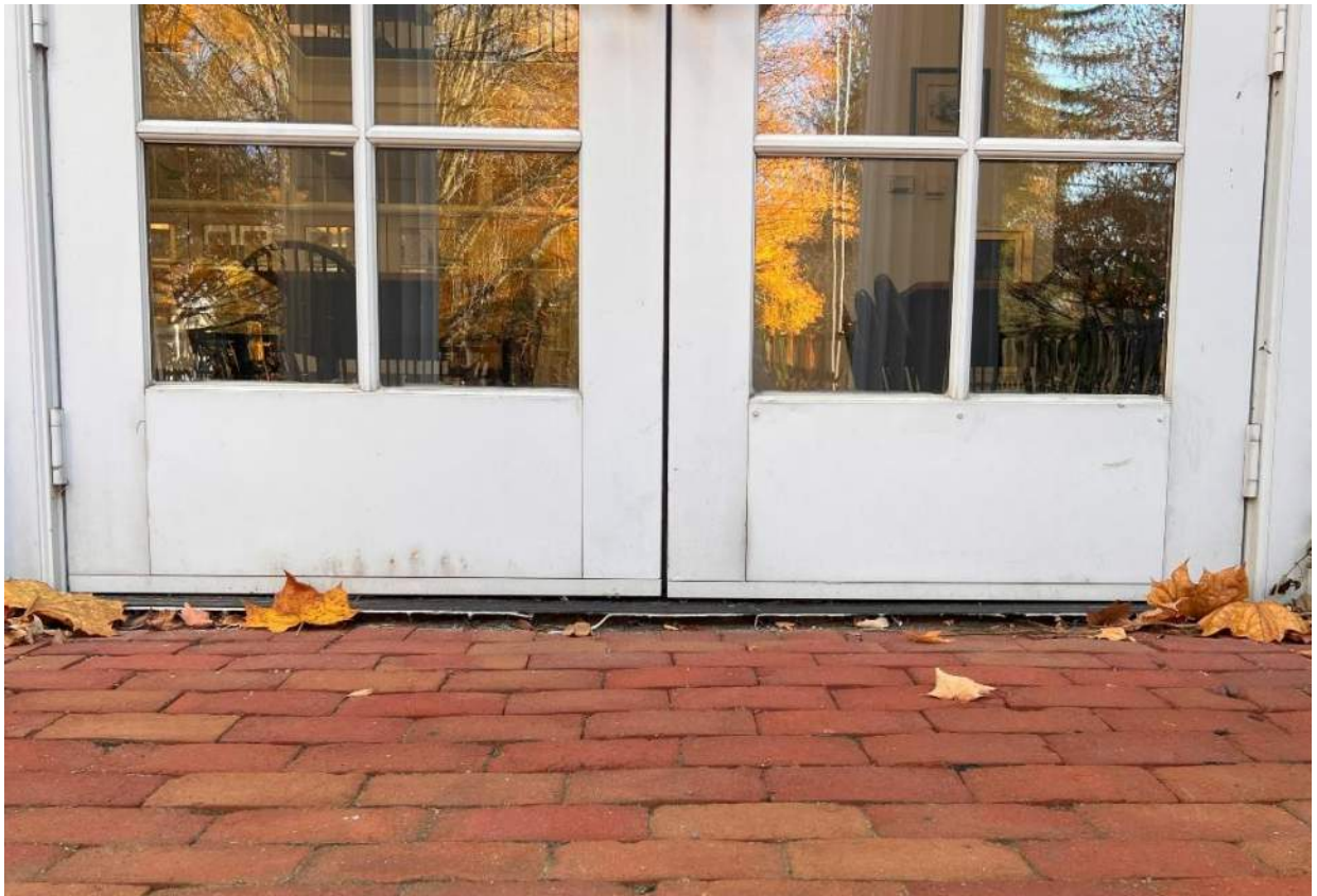
Figure 9: Egress doors at central patio. Note broken sill.
