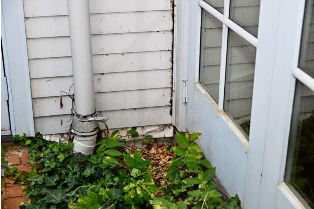
Figure 3: Northeast patio siding damage.
