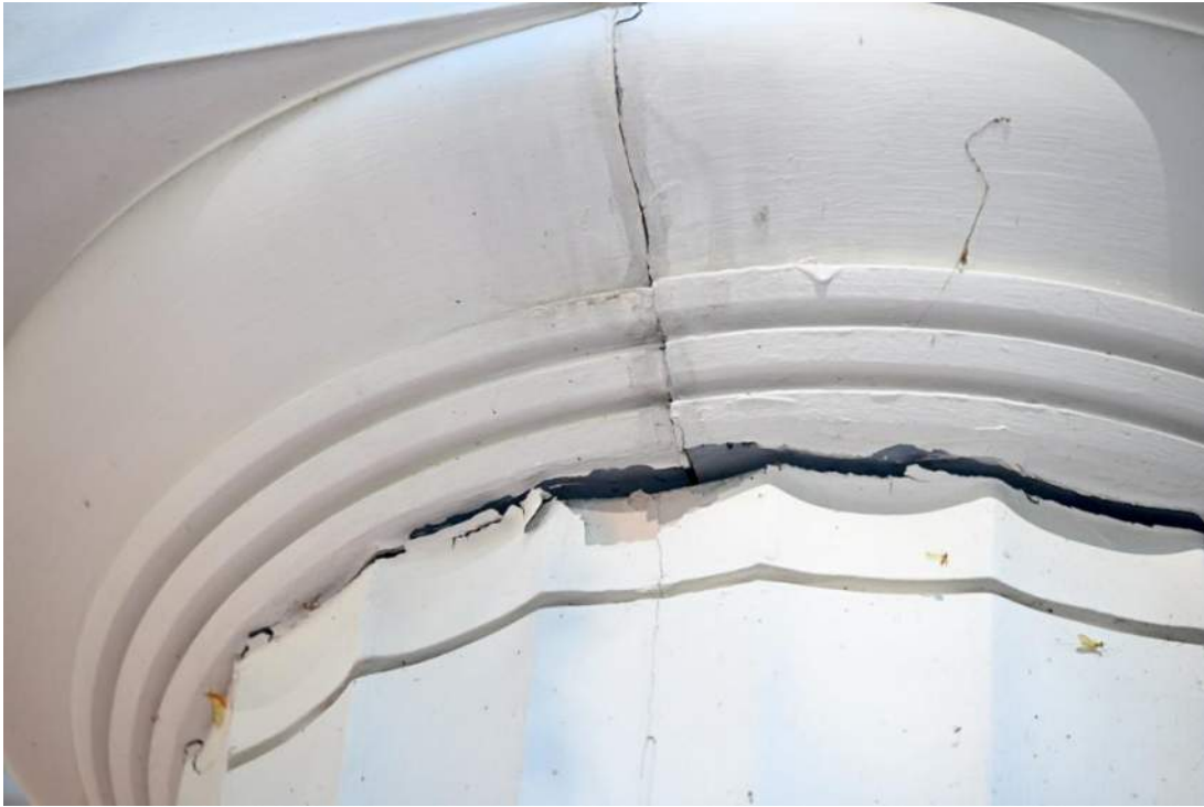
Figure 10: Crack in column capital.
