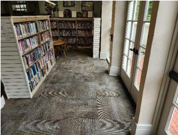
Photograph 16: Floor slab sloping in the Bookstore Area.
