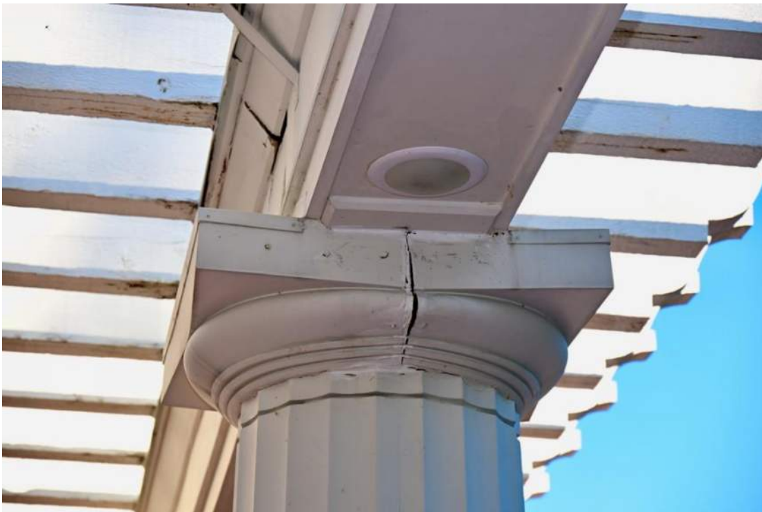
Figure 11: Major split at column capital near the parking lot.
