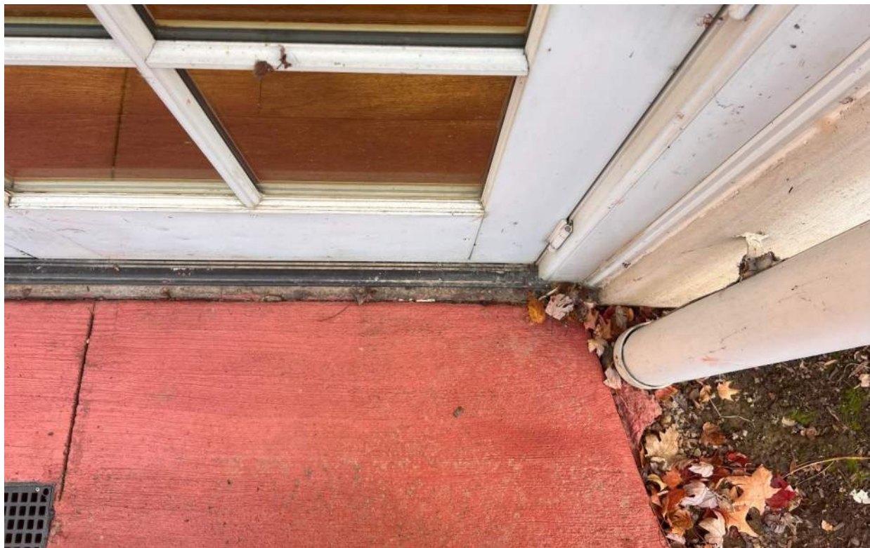
Figure 7: Active door sill at South Elevation.
