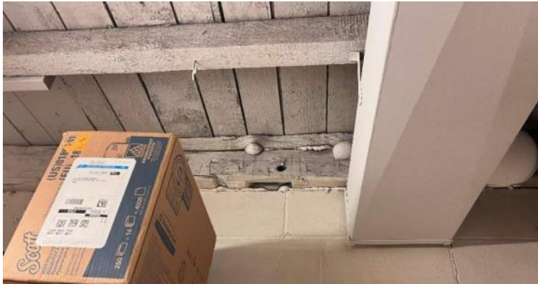
Figure 1: Foundation CMU wall and wood beam connection. Location of both wall and wood trim exposure.
