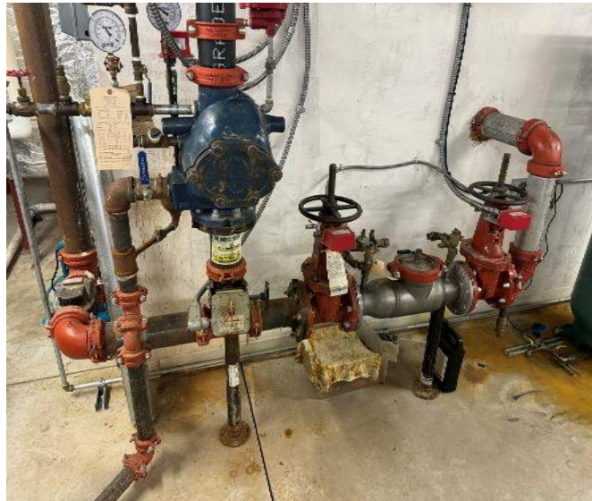
Fire Service and Riser
