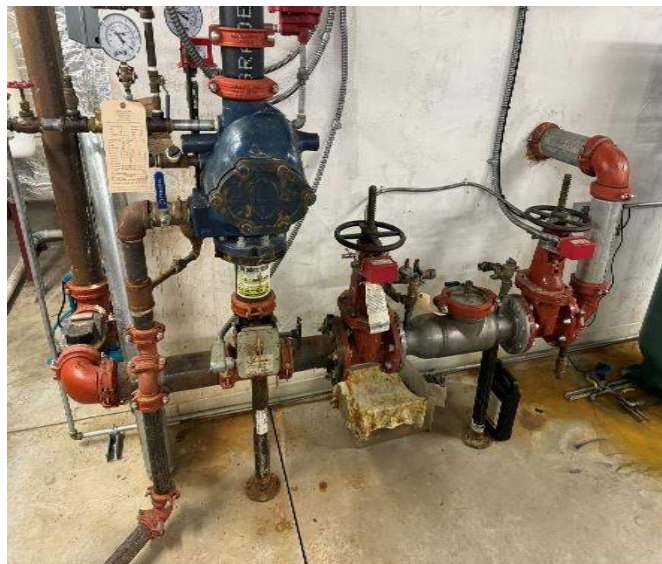
Photograph 17: Fire Service and Riser.
