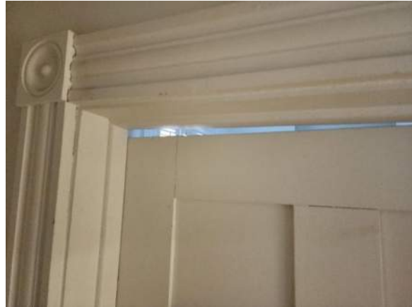
Photograph 19: Gap at door.
