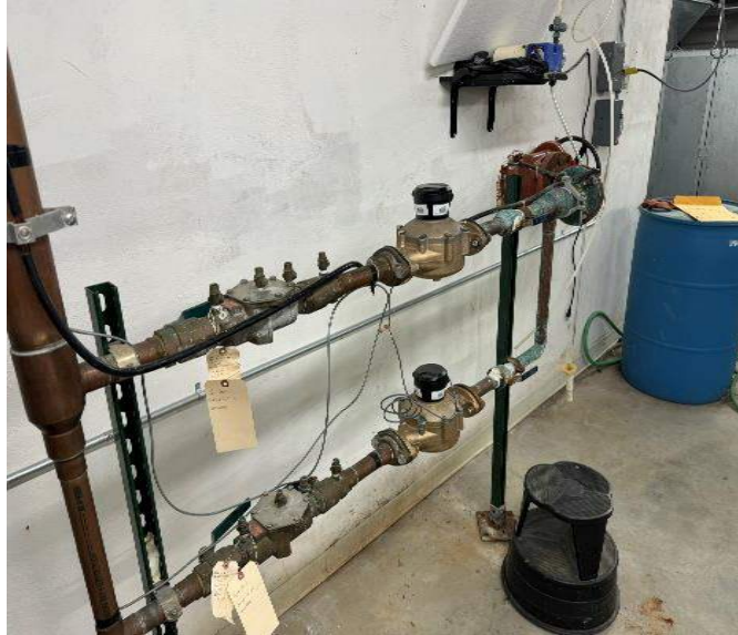
Photograph 11: Water Service Backflow Preventer.
