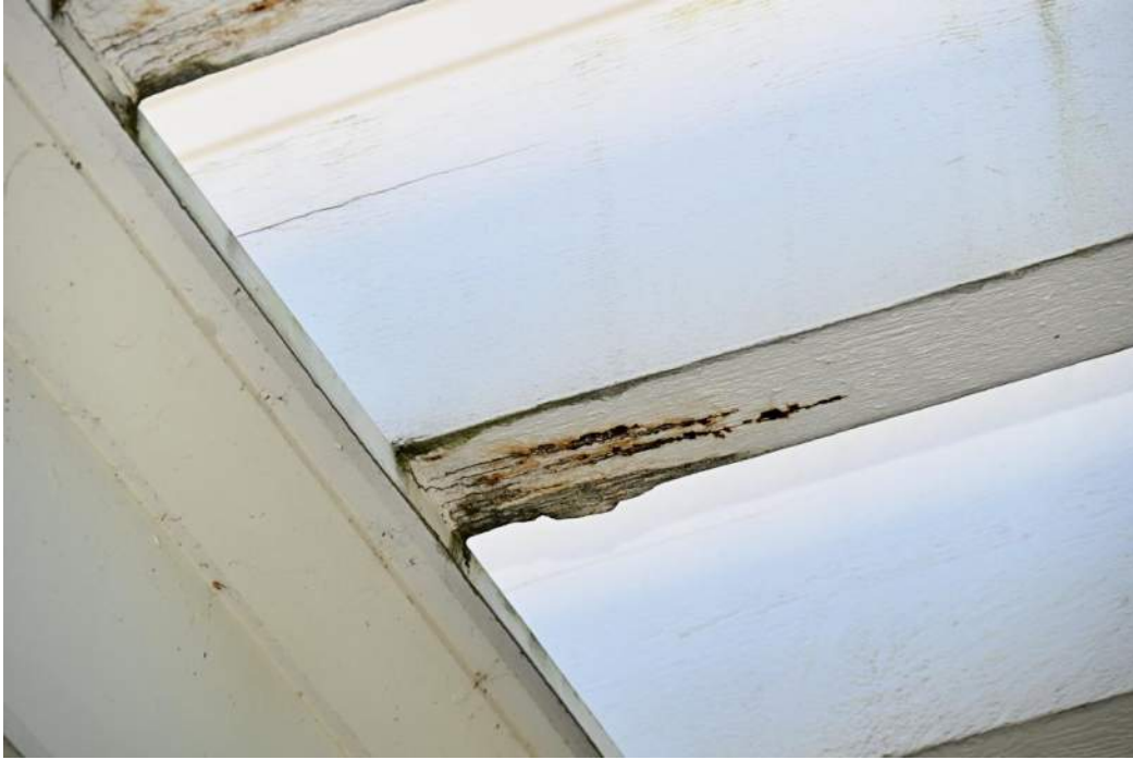
Figure 3: Pergola wood joists highlighting rot and metal trim beneath.
