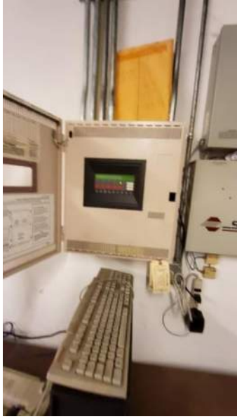
Photograph 27: Fire Alarm Control Panel.
