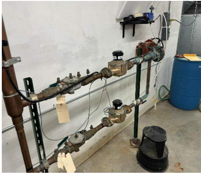
Water Service Backflow Preventer
