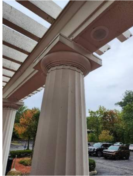
Photograph 8: Column wrap failure.
