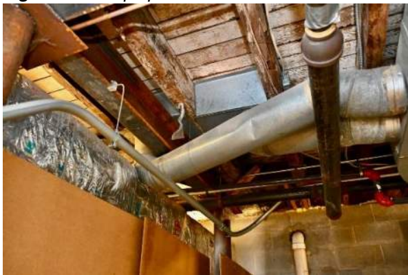
Figure 3: Lack of space beneath floor joists.
