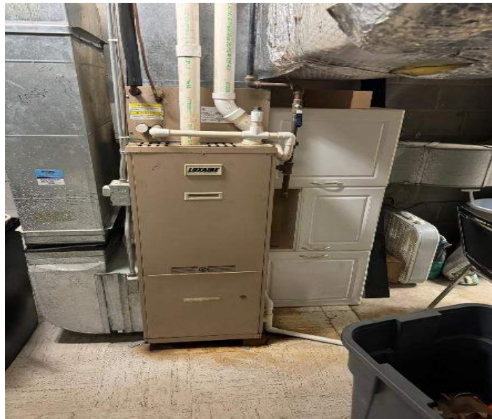
Furnace/AC Unit (original building)
