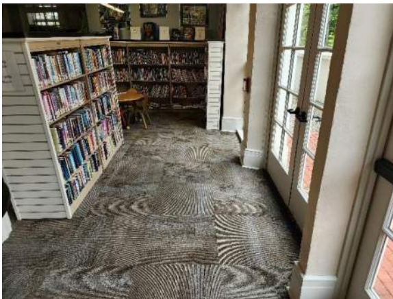
Photograph 13: Floor slab sloping in the Bookstore Area.
