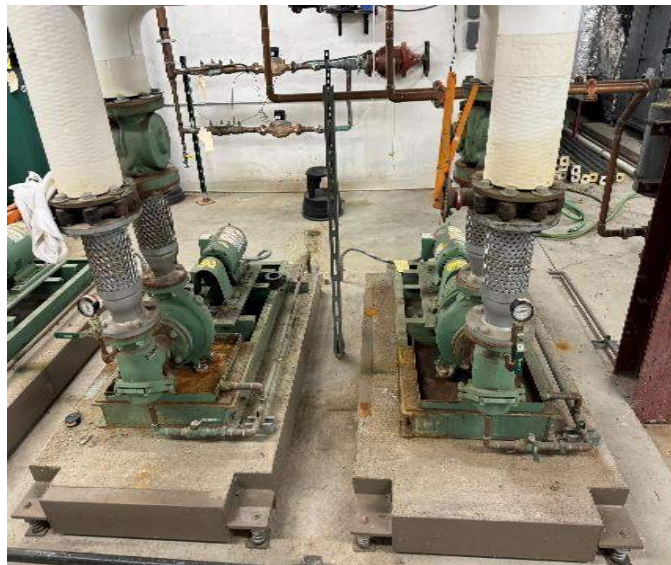
2- Hot Water Pumps
