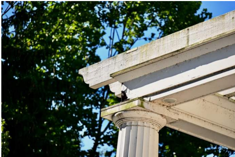
Figure 9: Pergola corner condition near parking lot.
