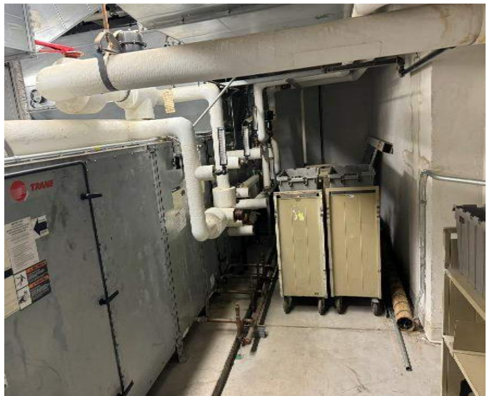
Photograph 6: Indoor Air Handling
