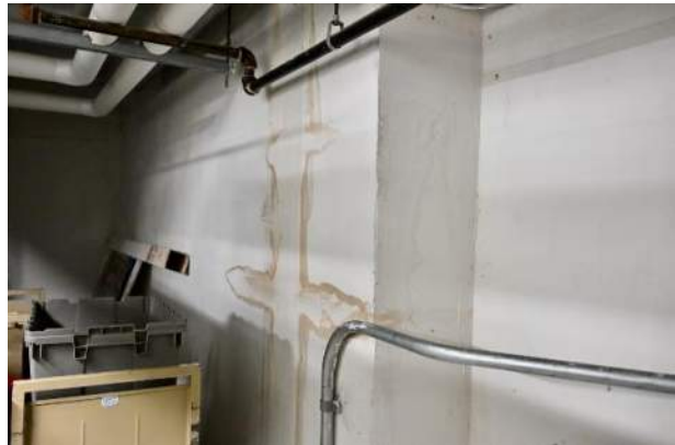
Figure 2: Discoloration of West basement wall.
