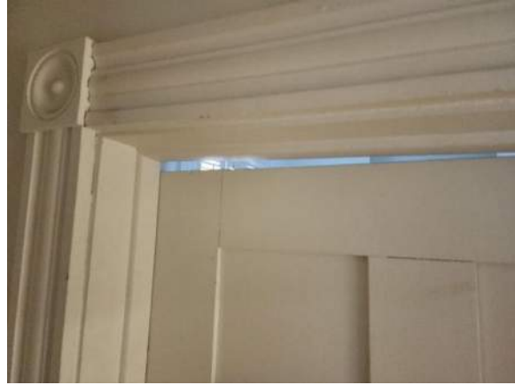
Photograph 24: Gap at door.
