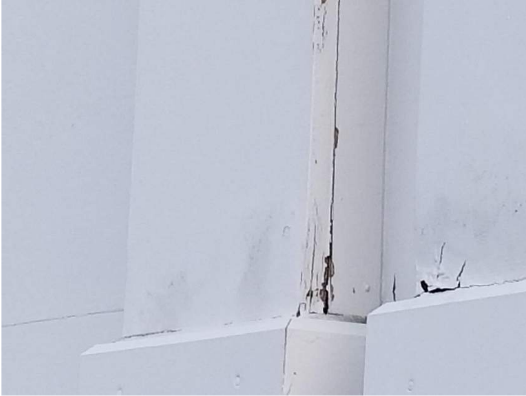
Figure 18: Cupola pilaster cracks from rot.
