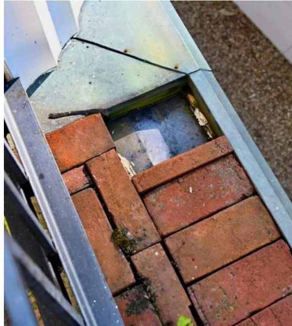
Figure 2: Northeast Balcony shows missing pavers and moss growth.
