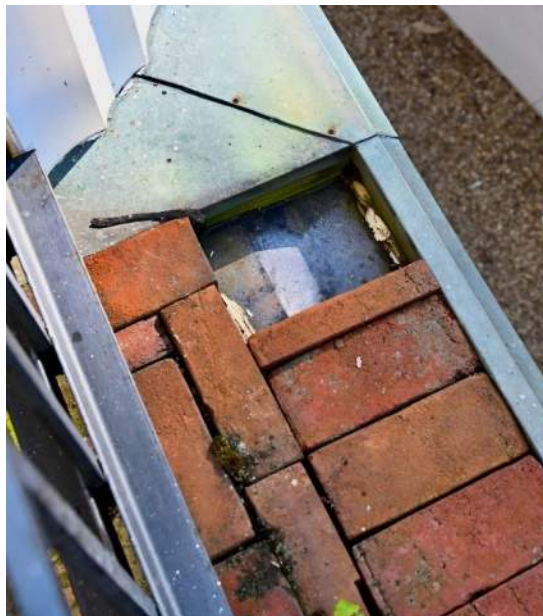
Figure 2: Exposed membrane at the balcony facing the parking lot.
