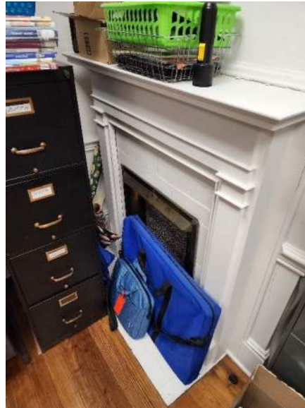
Photograph 22: Cracking around fireplace.
