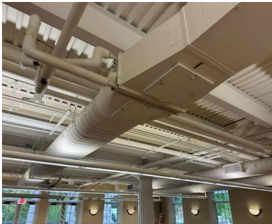
Photograph 7: Space Reheat Coil.
