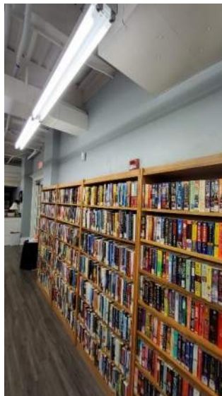
Photograph 25: Stack Area Lighting.
