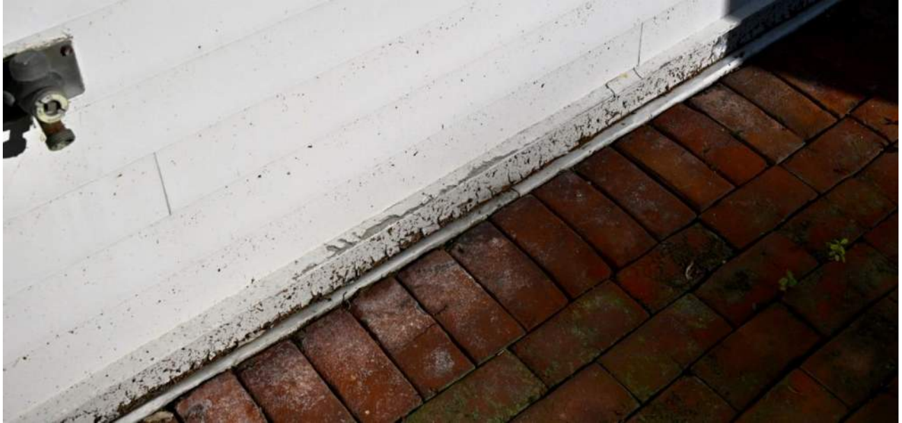
Figure 1: Condition of the trim on the Southern balcony.
