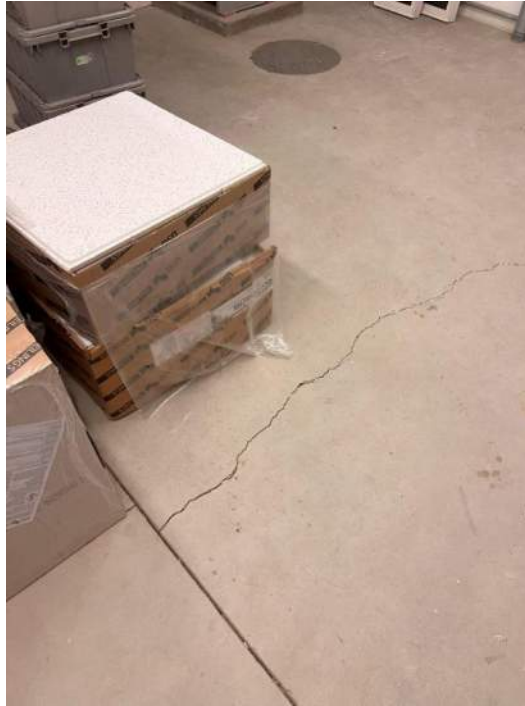
Photograph 15: Crack shown in floor slab.
