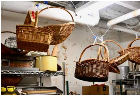
Figure 1: Damp spots on the West wall.
