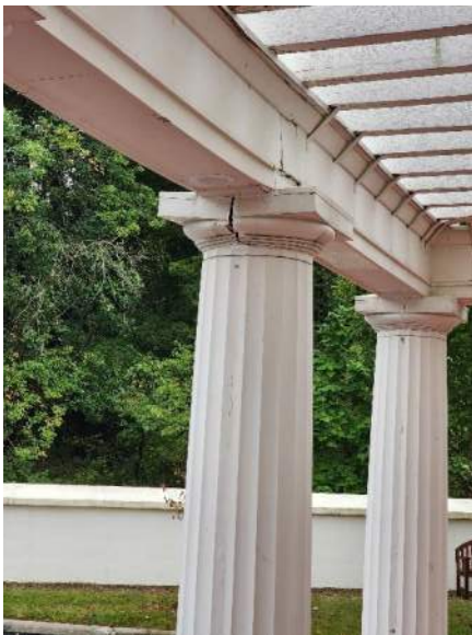
Photograph 7: Column wrap failure.
