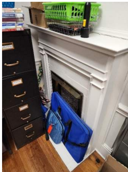
Photograph 17: Cracking around fireplace.
