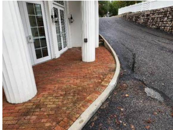
Photograph 5: Absent frost slab at outswinging exterior door.
