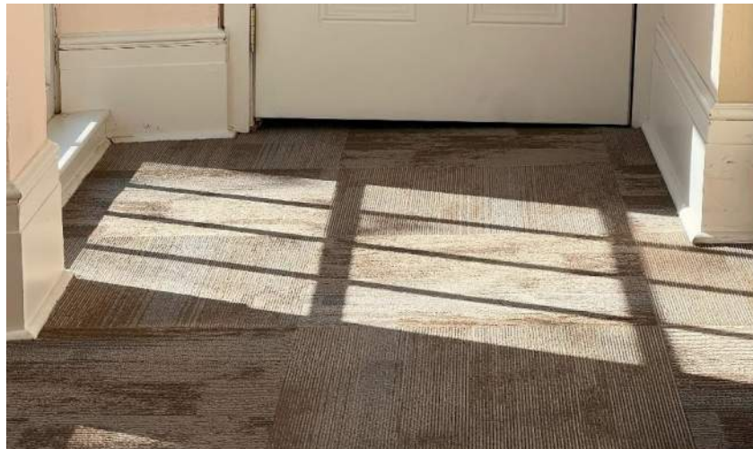
Figure 2: Book Store slab settlement issues.
