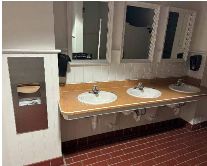
Photograph 14: Lavatories w/Manual Faucets.
