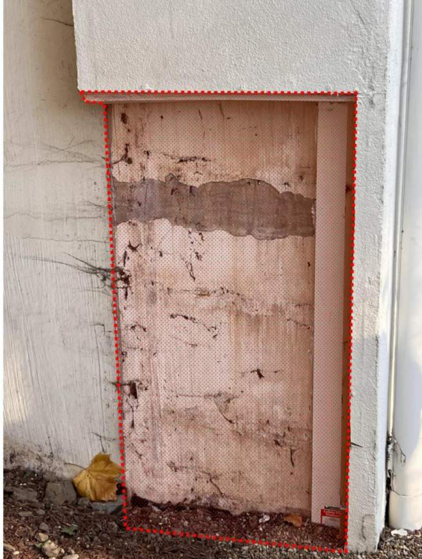
Figure 12: Concrete exposure on West Elevation. Red hatch shows desired infill.
