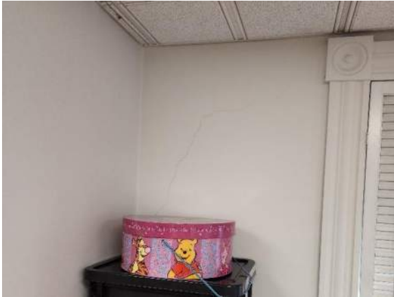
Photograph 18: Cracking in wall.
