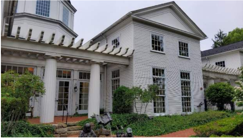
Photograph 26: Exterior Wall Lights and Façade Lighting.
