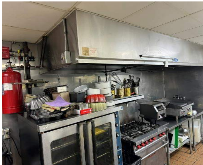
Photograph 19: Type 1 Kitchen Hood.
