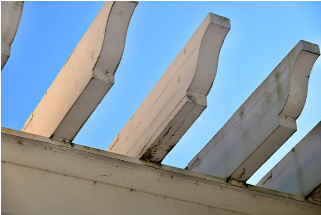
Figure 4: Pergola wood joist resting on beam. Notice weathering and decay of wood members.
