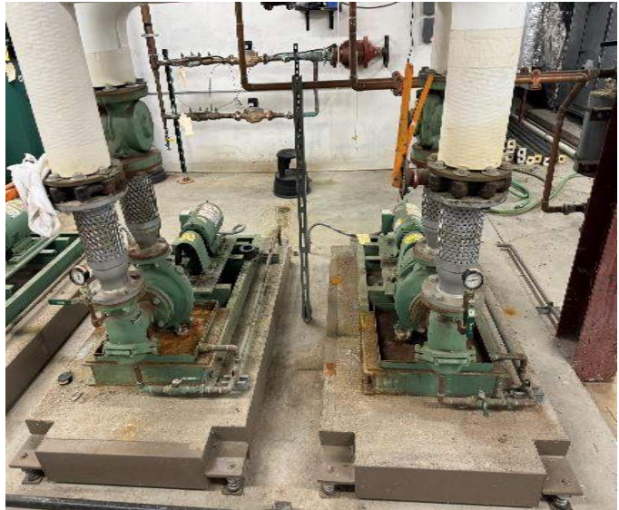
Photograph 5: Hot Water Pumps.
