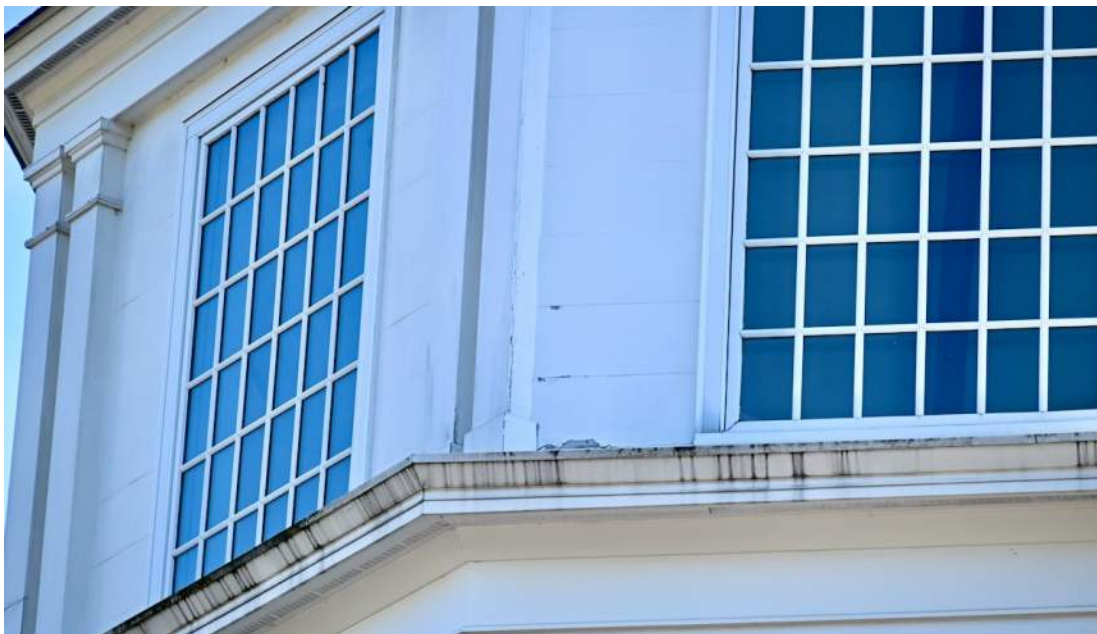
Figure 19: Center cupola trim and pilaster issues.
