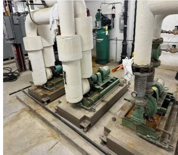
Photograph 10: Chilled Water Pumps Coil.
