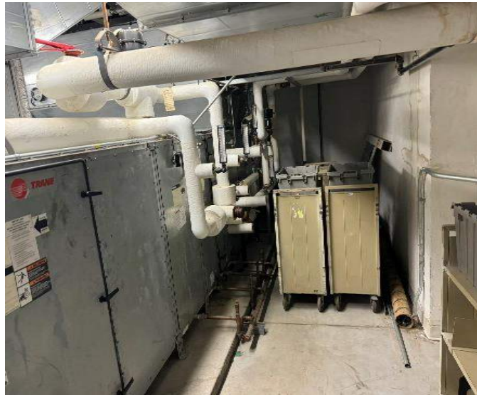
Indoor Air Handling Unit
