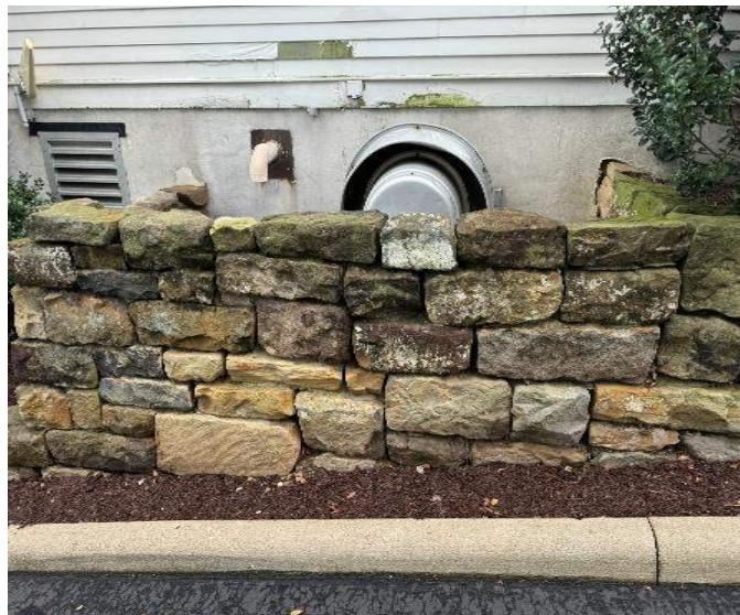
Kitchen EF Discharge
