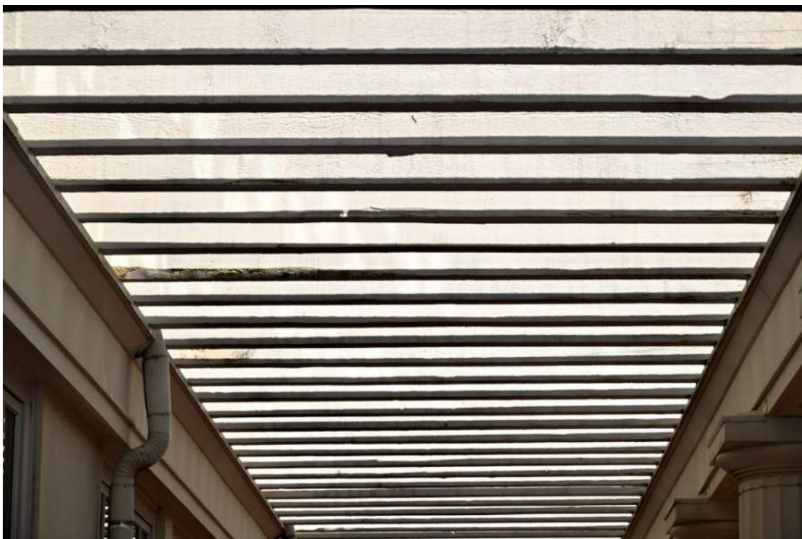
Figure 13: Joist deterioration at South Elevation.
