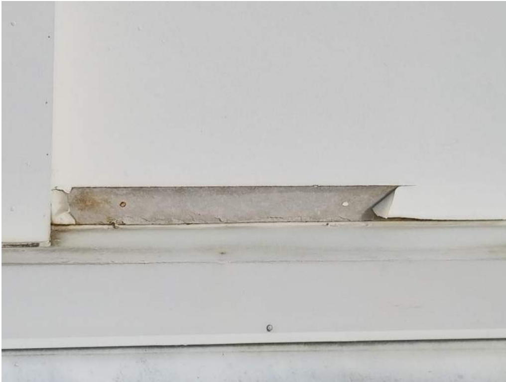
Figure 15: Cupola trim peeling at base.
