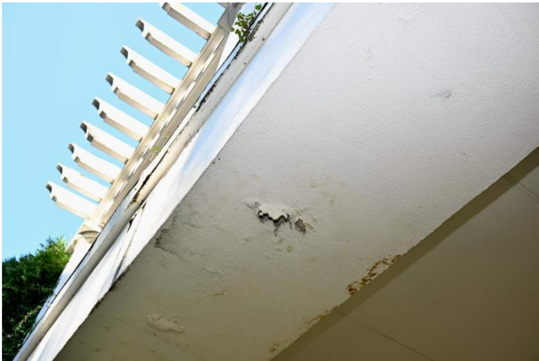
Figure 4: EFIS damage underneath the main-level balcony.
