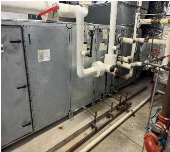
Photograph 9: AHU with Chilled Water Coil.
