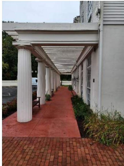
Photograph 6: East sidewalk slopes toward building.
