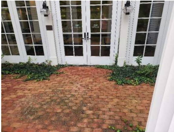
Photograph 4: Absent frost slab at outswinging exterior door.
