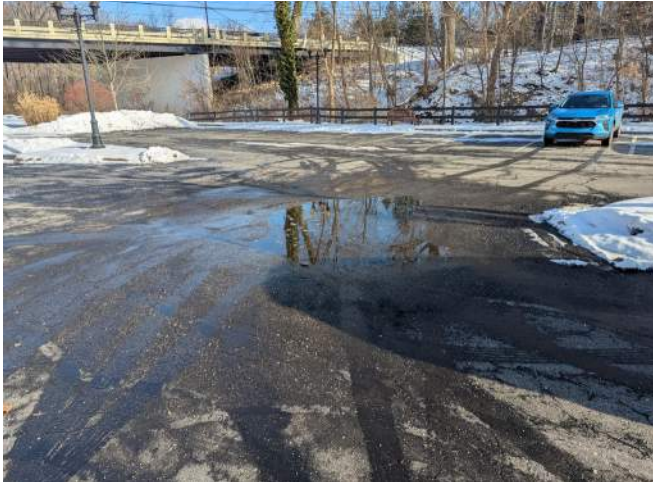
Figure S-2: Ponding water in parking lot
