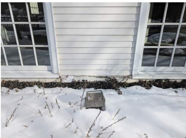
Figure A-3: Deteriorating siding
