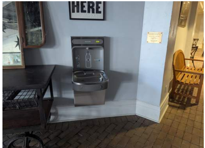
Figure A-15: Drinking fountain
