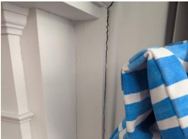
Figure A-21: Fireplace crack in dormitory building
