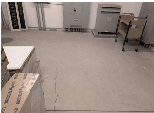
Figure A-25: Cracked floor in electrical room
