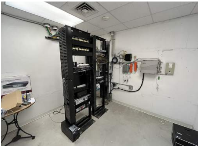
Figure E-2: Floor mounted IT rack
