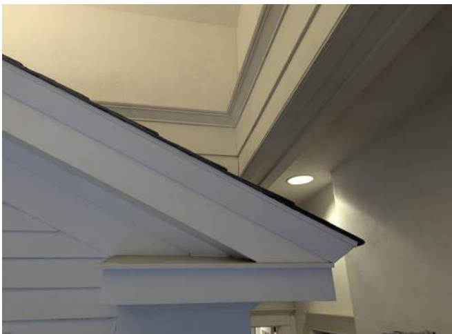
Figure A-23: Crack in corner of moldings
