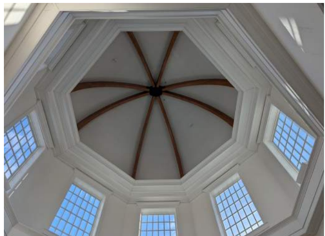
Figure A-24: Water stains on cupola ceiling
