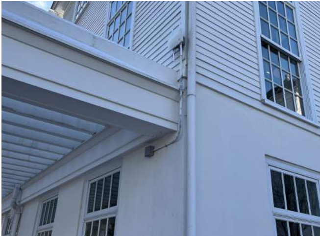
Figure E-6: Exterior wall mounted wireless access point
