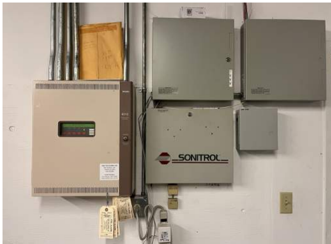
Figure E-1: Fire alarm control panel
