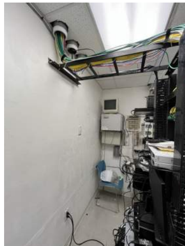
Figure E-3: Technology wiring in IT room
