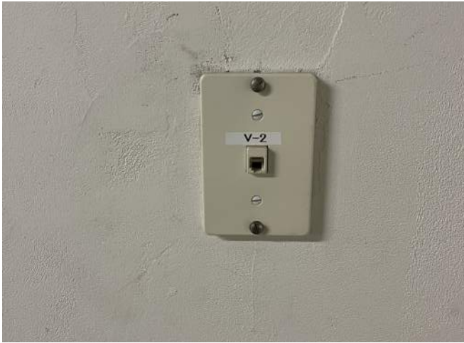
Figure E-4: Data receptacle
