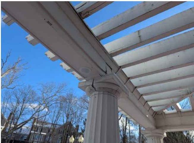
Figure A-1: Failing pergola column and beam
