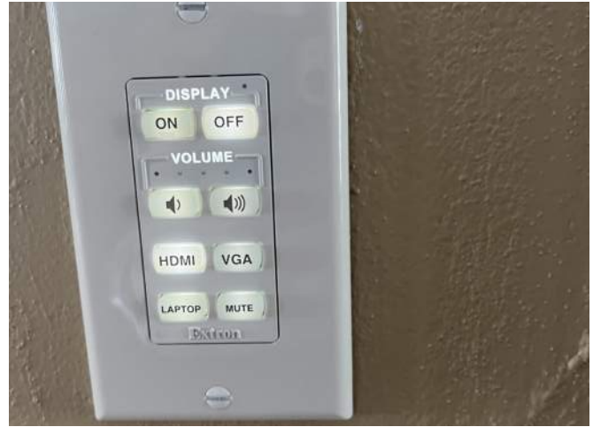
Figure E-5: Presentation controls in meeting room
