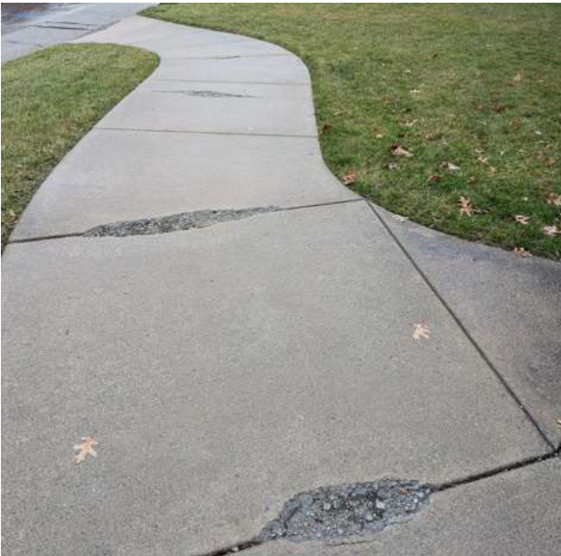
Damage to internal site sidewalk
