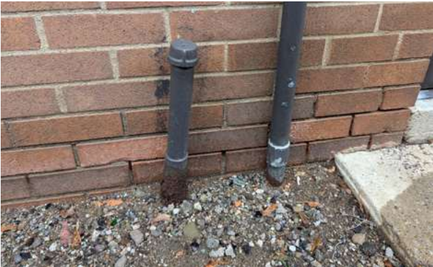
Masonry condition at base of wall; corroded metal pipe
