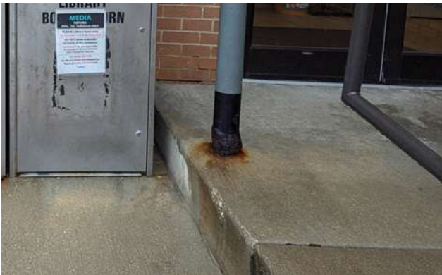
Corroded metal pipe at parking lot entry near exterior book drop
